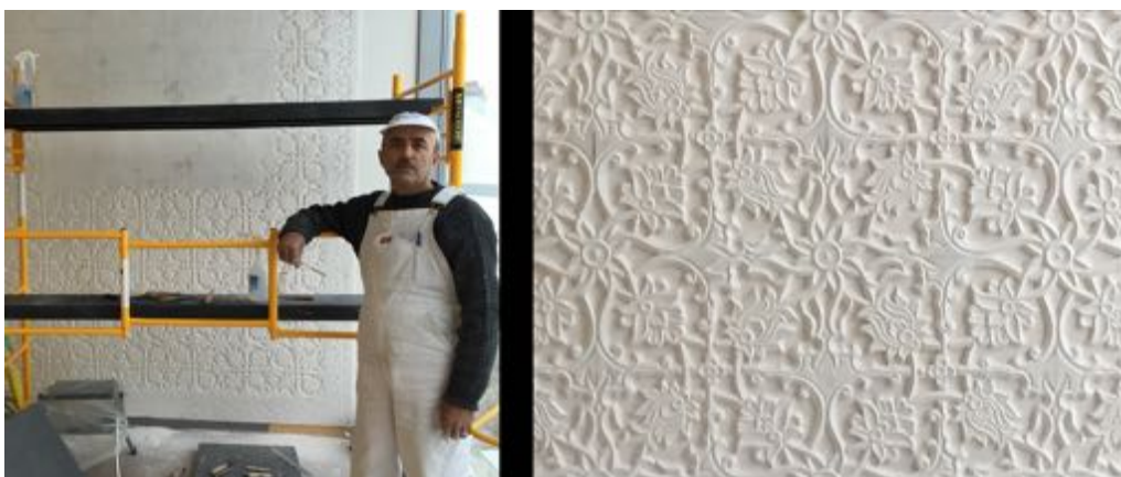
Figure 9.25: White plaster wall with arabesque design by master artisan from Tajikistan Credit: Hussein Charania
