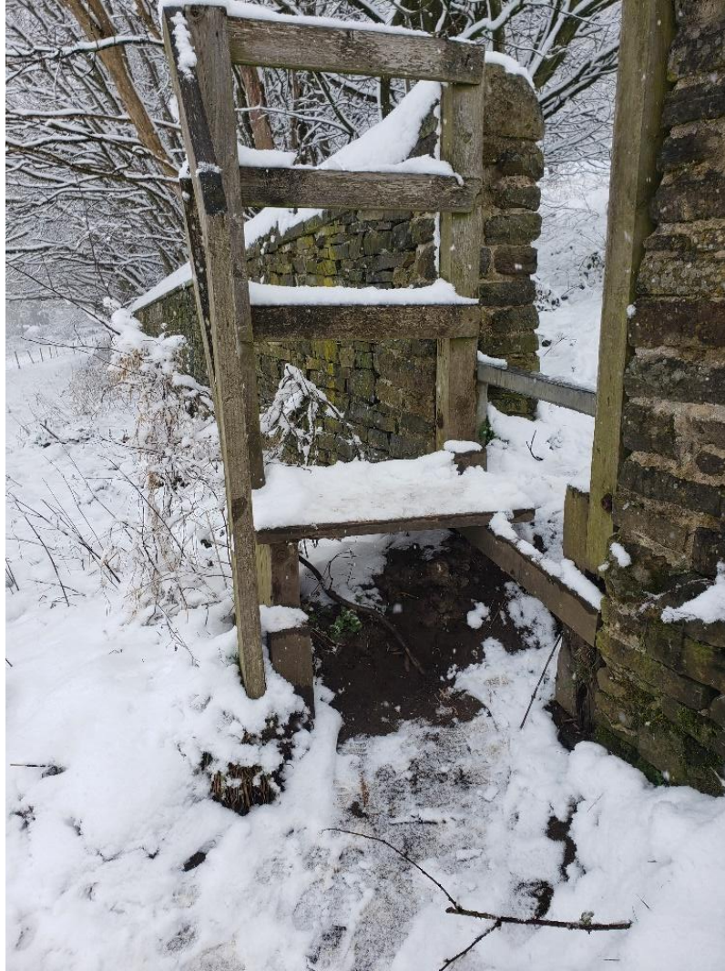
Image 4: A missing step on a footpath stile with snow (A. Flint)
